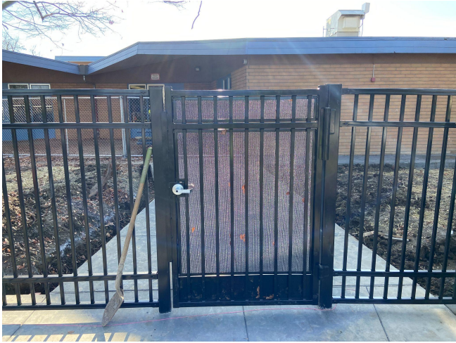
Security Fencing Multiple Sites
