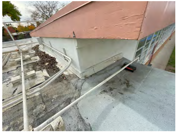
Example of the metal flashing at the transition between the roof and stucco. Asbestos containing black mastic was found between the flashing and stucco.
