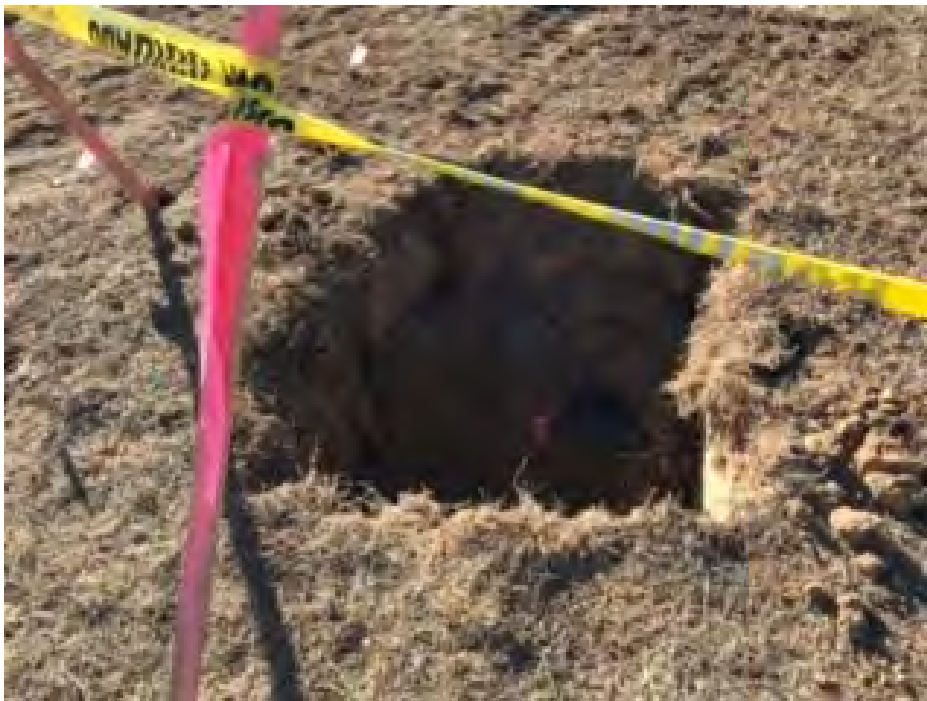
Initial limits of excavation activity on October 25, 2023 later expanded on November 6 and November 20, 2023.
